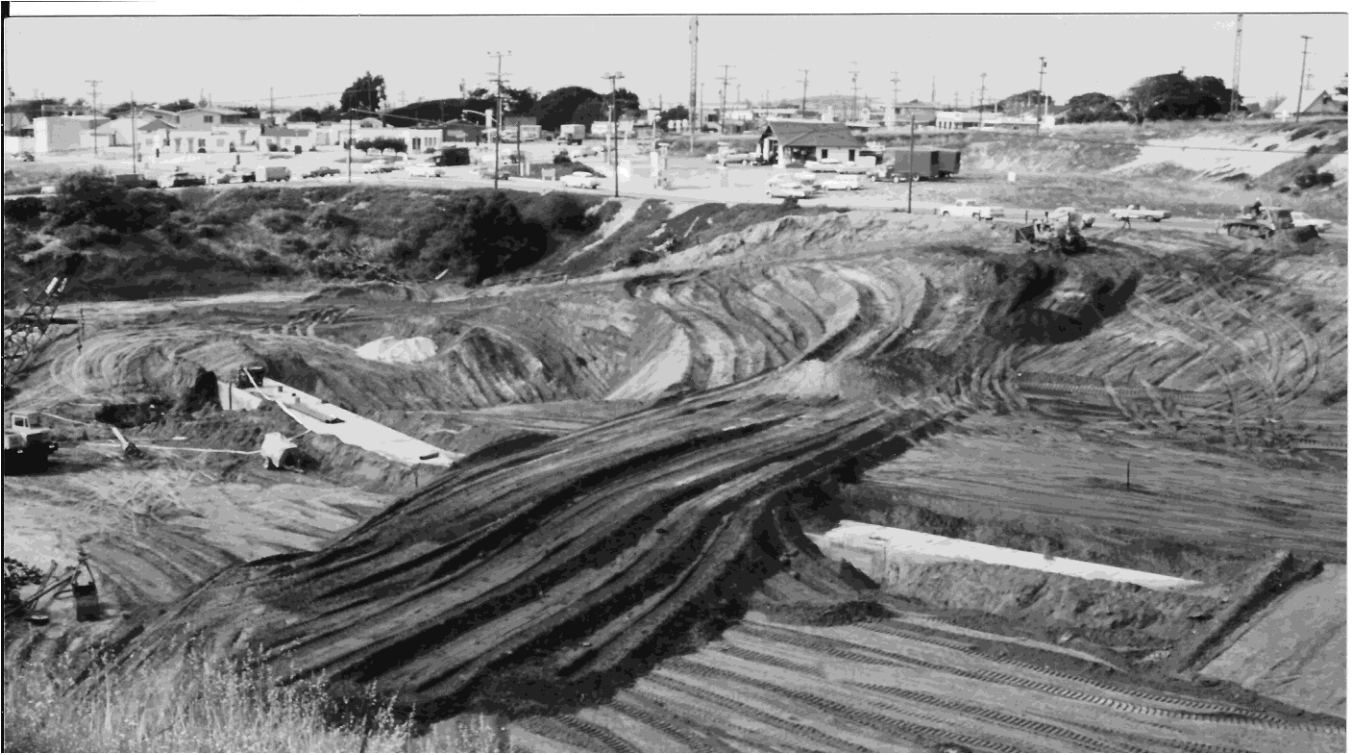
Photographic view of the present Safeway site, N. Fremont/Canyon Del Rey intersection (Walgreens is now in the upper left of photo). In view is a concrete culvert that collects the creek water from Del Rey Oaks and routes it to Laguna Grande Lake. This photo shows the start of filling of the canyon with over 16,000 truckloads of soil. The original store (MonteMart) was completed 8 months later for a total cost of $2.5 million dollars. A included Herald article gave the above information c1966.....Photo is donated from the estate of Dick Bowman, photo taken from his backyard on Melway Circle.
